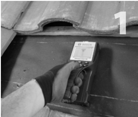
1 Remove the tile at selected location of the mount. Locate and mark the center of the rafter.
